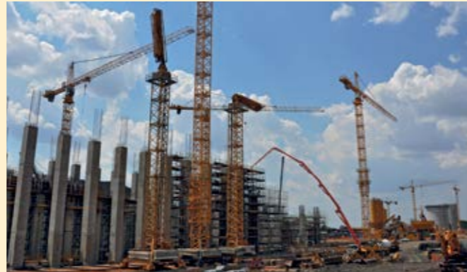
2011 2 x MX 47 were used for the Madupi Power station project in Limpopo Province .
