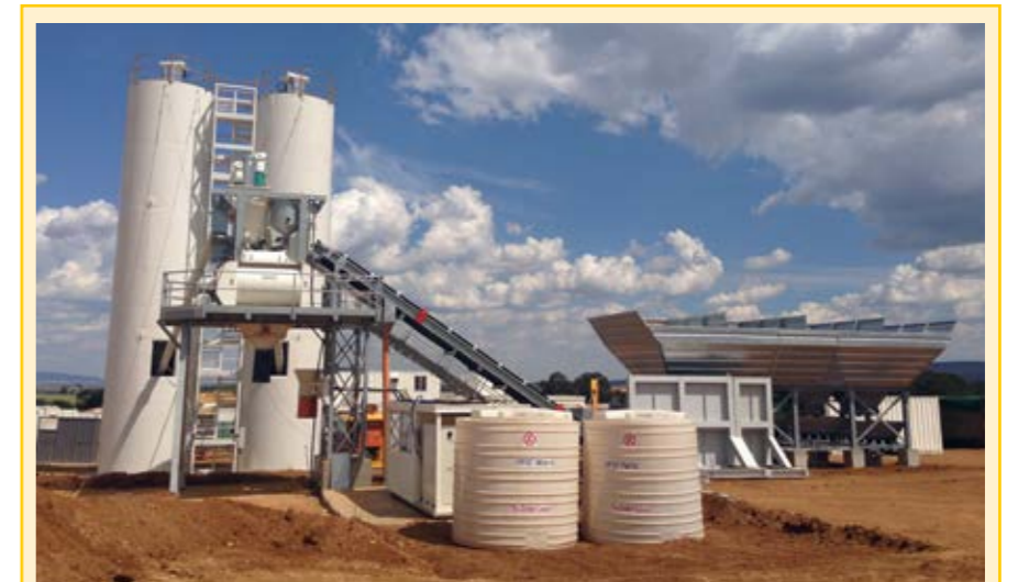
Simem Eagle 4000 mixing plant:
