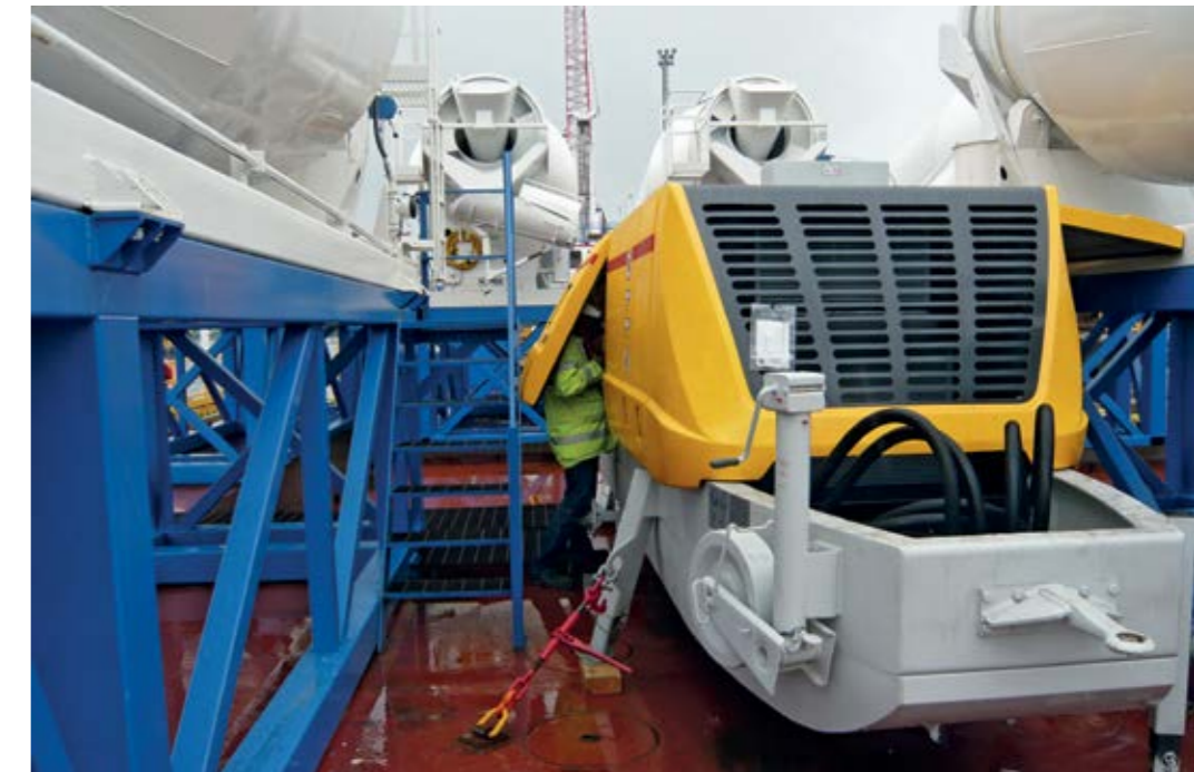
▲ A stationary concrete pump BSA 2110 HP D is loaded by the six truck mixer drums and delivers the concrete to a truck-mounted concrete pump or a stationary boom on the barge.
