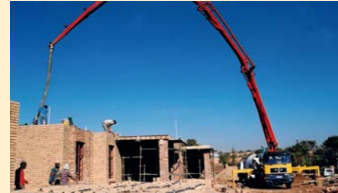
2003 This BSF 32.09 was used for a housing project in Johannesburg, South Africa
