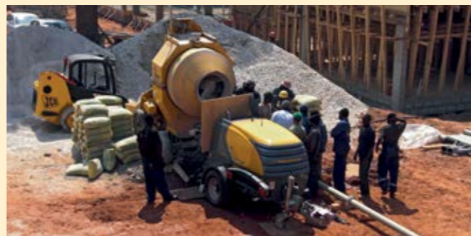
2011 A fine concrete pump P 715 was used for the Lusaka Housing Estate project in Lusaka, Zambia
