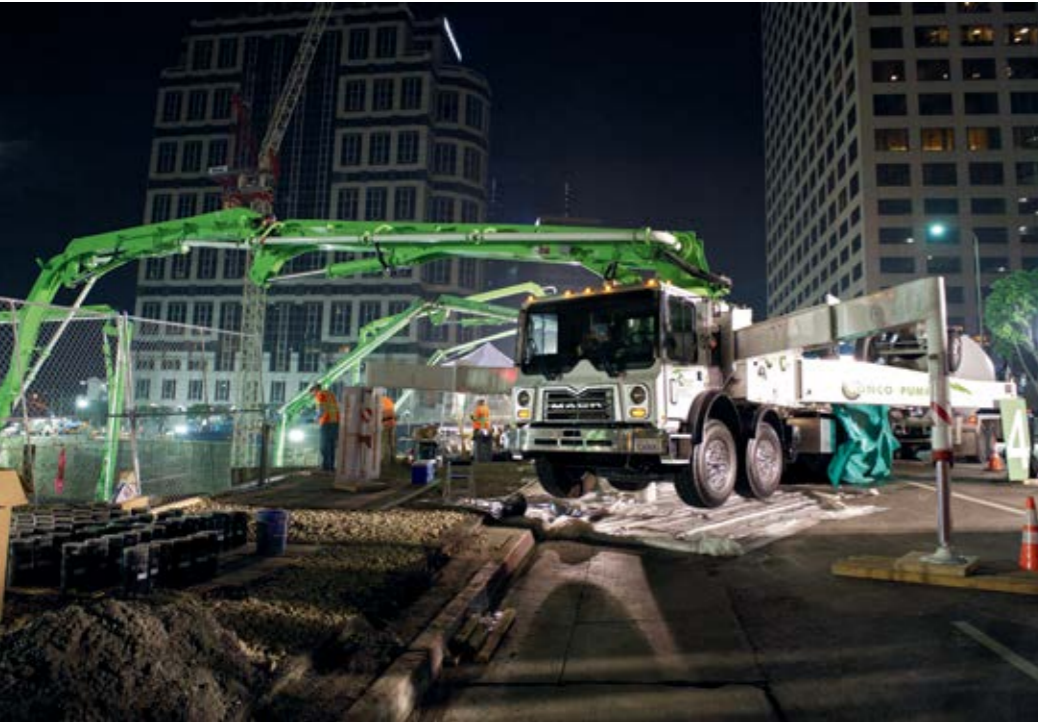
▲ In order to minimise interferences for businesses and residents, the concreting work started on Saturday evening and was completed on Sunday at midday.
