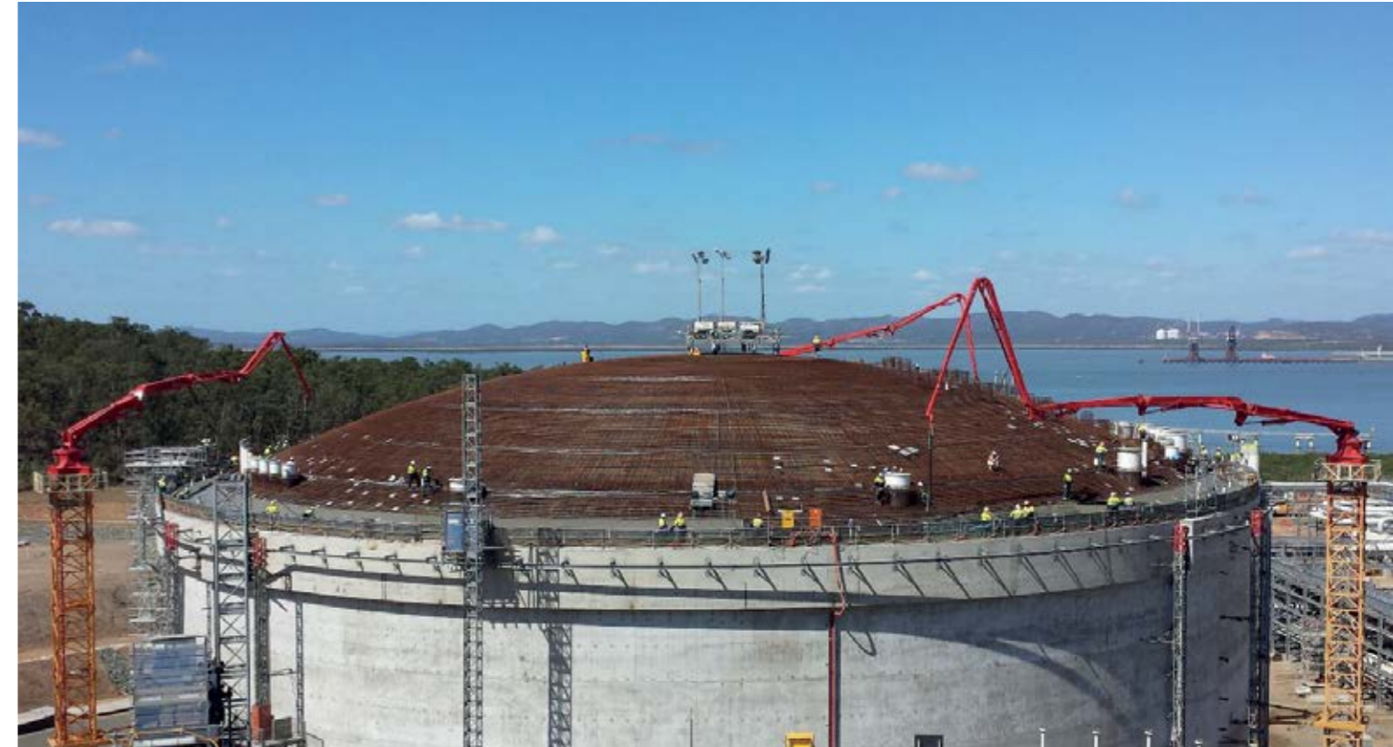
▲ The project is using six MX 43-5 placing booms mounted on 40 m high freestanding lattice tower sections, and two M 47-5 pumps to assist larger pours.
