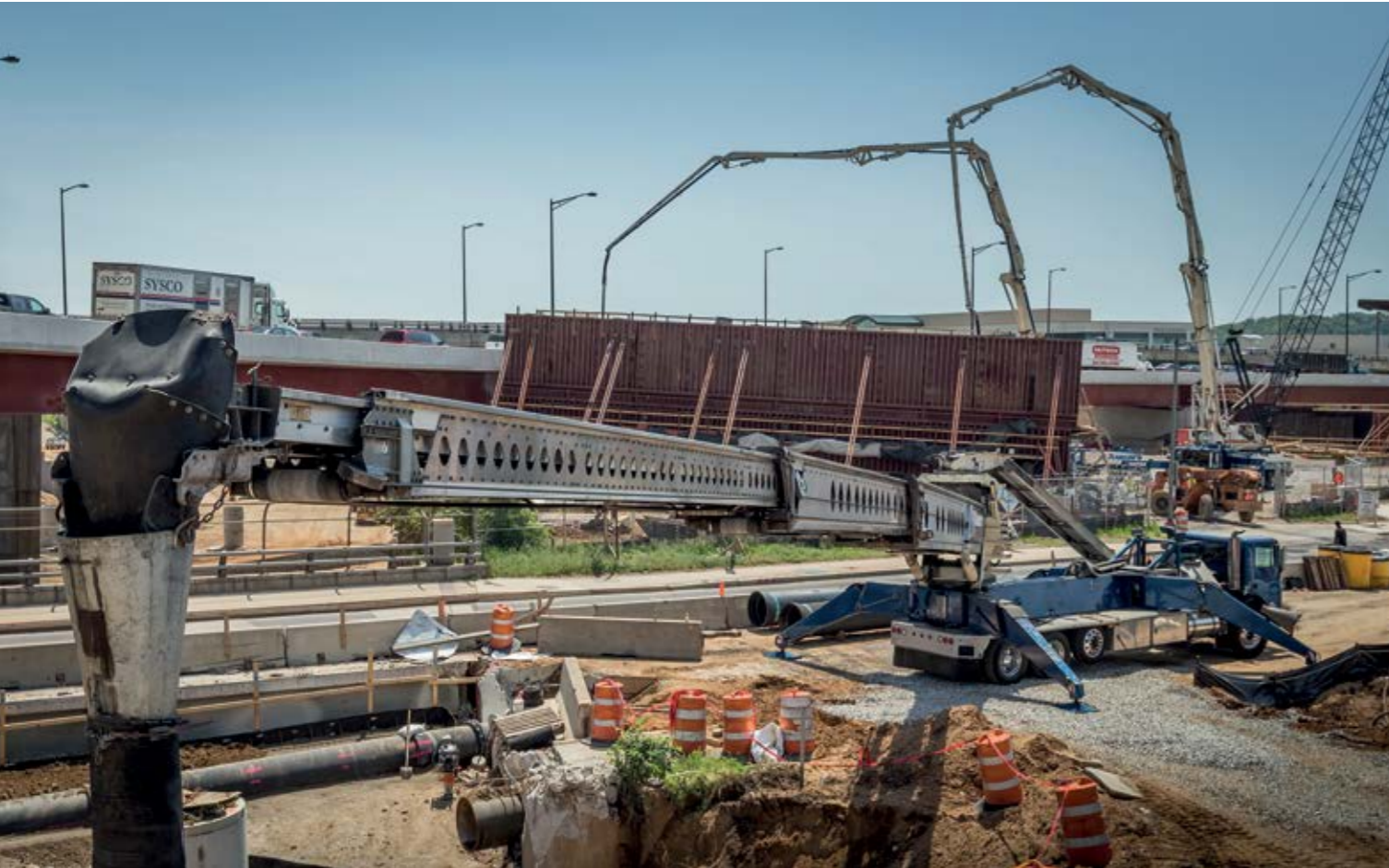
▲ A Putzmeister Telebelt TB 110 is being used to place the stone and dirt for the bridge abutments.
