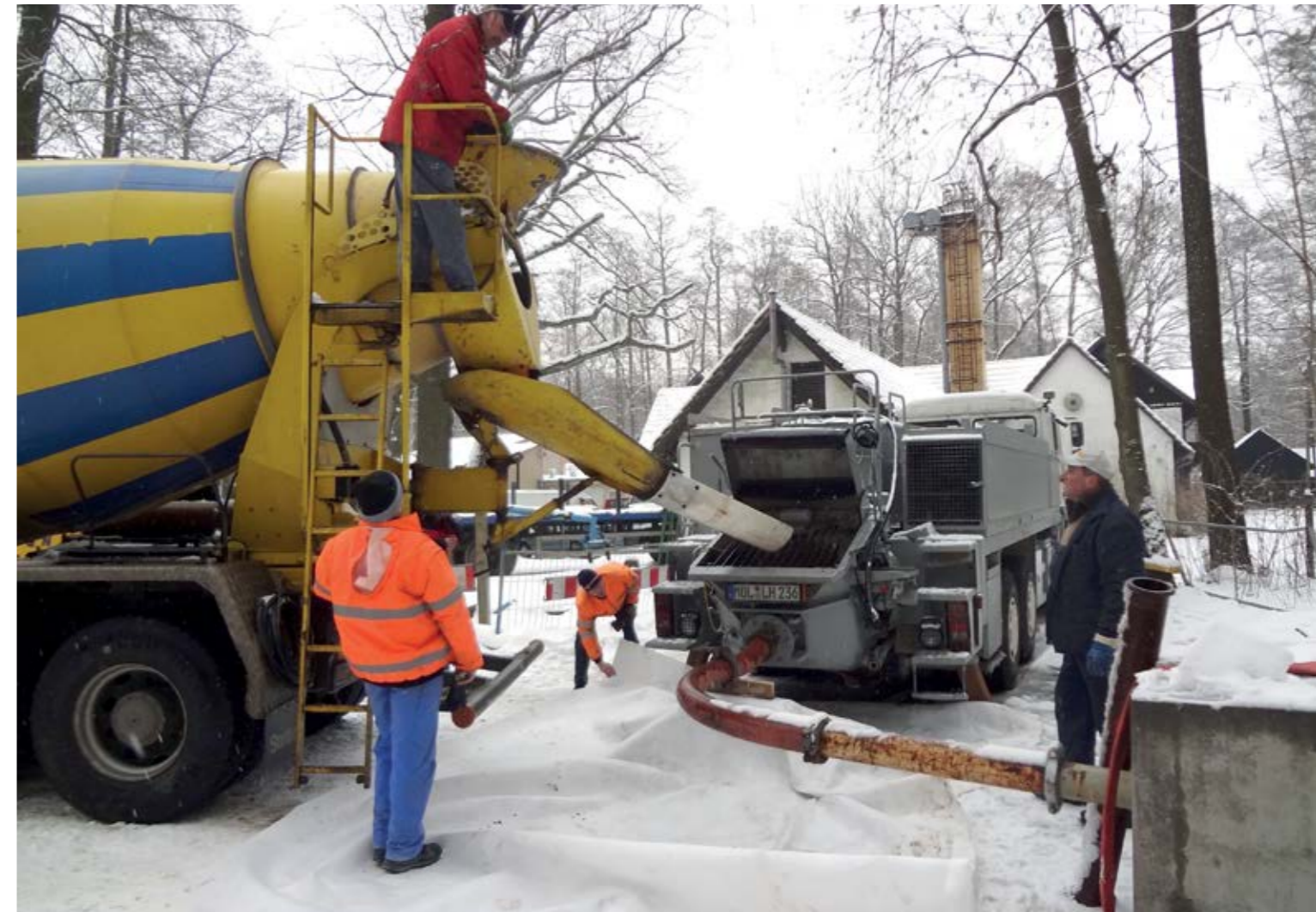
▲ The Moli 21.12 pumps material along the 450m pipeline. The pipeline is secured in position with a heavy concrete block.
