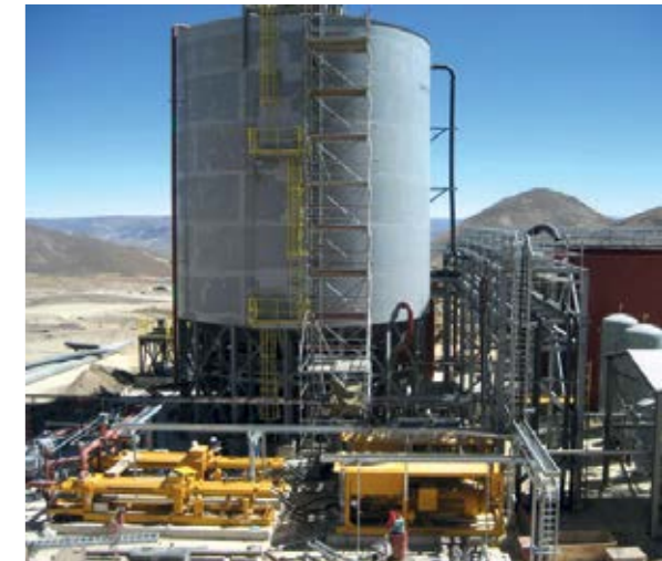
▲ Backfilling pump system under a paste thickener constructed on the San Bartolome silver mine in Bolivia
