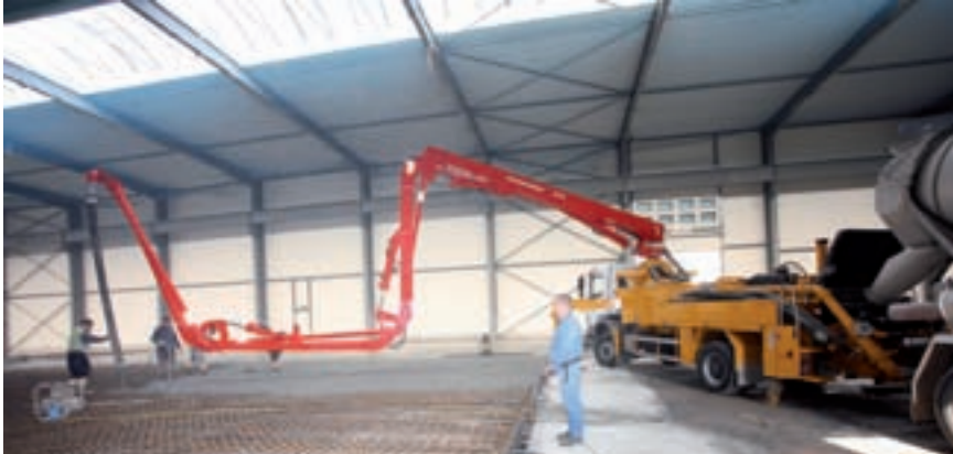
Superior performance when concreting in low buildings – thanks to low unfolding height and flexible roll-Z-fold system
