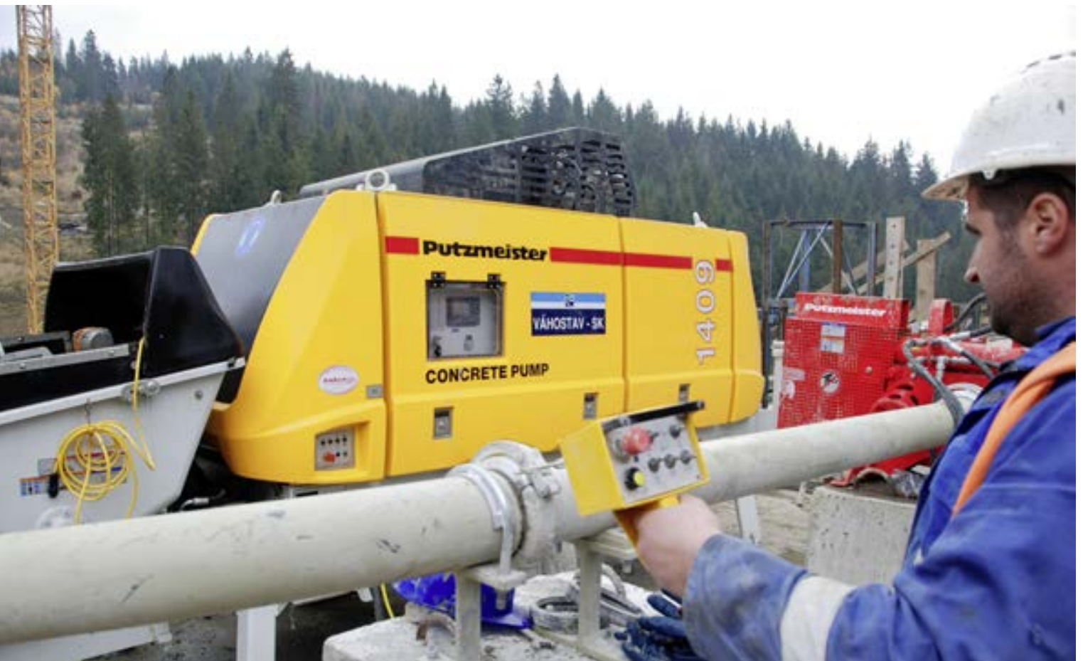
The gate valve is hydraulically driven and controlled by the stationary pump
